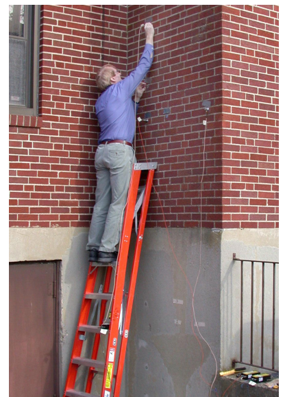
Our tests involved placing vibration sensors on the exterior of a building. Vibration sources were placed at several locations within the building.
